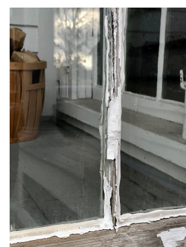
Close up of damage
