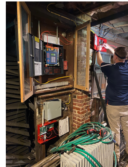
Fire alarm system
