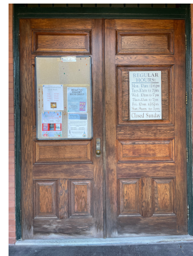
Close up of damage
