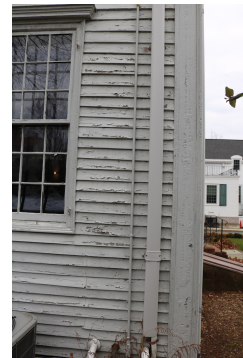
Close up of damage
