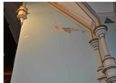
Interior water damage
