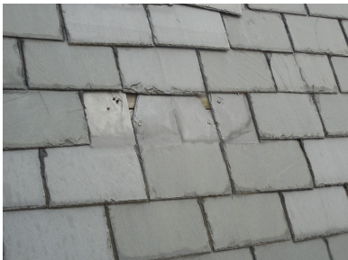
Roof slate damage
