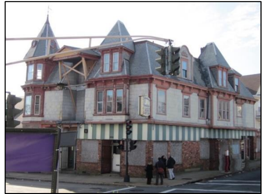
Oscar Romero House in New Bedford was vacant for over 15 years and in deplorable condition before its renovation
